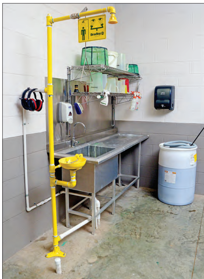
Eye wash station. Credit: J. Brosnan.
