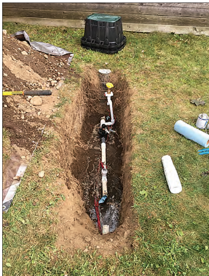
Master valve and flow sensor installation. Credit: B. Polimer.
