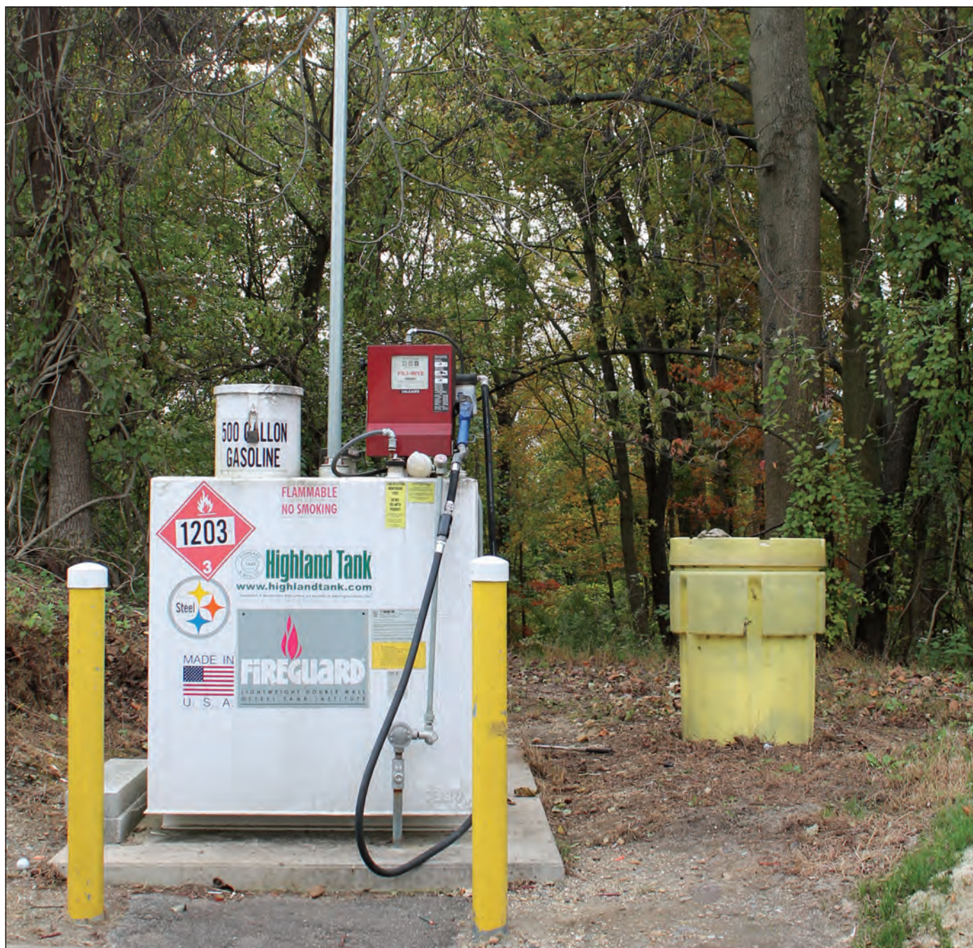
Fueling area. Credit: S. Kingsbury.
