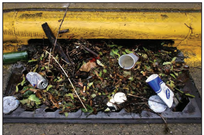
Grates can filter trash and debris from stormwater - Picture courtesy of Aaron Volkening, P.E.
